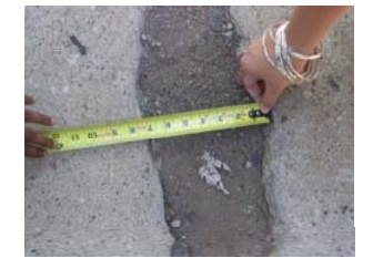
Cracked Sidewalk within Project Site: a common problem the senior citizens face
